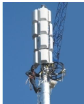
Weimar gets digital TV: In support of Germany's digital TV switch-over, Radio Frequency Systems (RFS) designed and installed a broadband panel antenna/combiner system for the rural German city of Weimar. The RFS system is a component of a 12-programme/three-channel DTV solution provided by one of Europe's major broadcast infrastructure groups. The combined terrestrial broadcast system provides DTV coverage to metropolitan Weimar and its surrounds.
